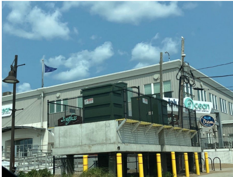
Figure 24: Elevated pad-mounted equipment in Salisbury, MA
