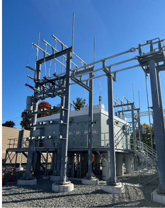
Figure 22: Substation equipment in Lowell, MA raised 6.5' above grade as a flood mitigation measure.
