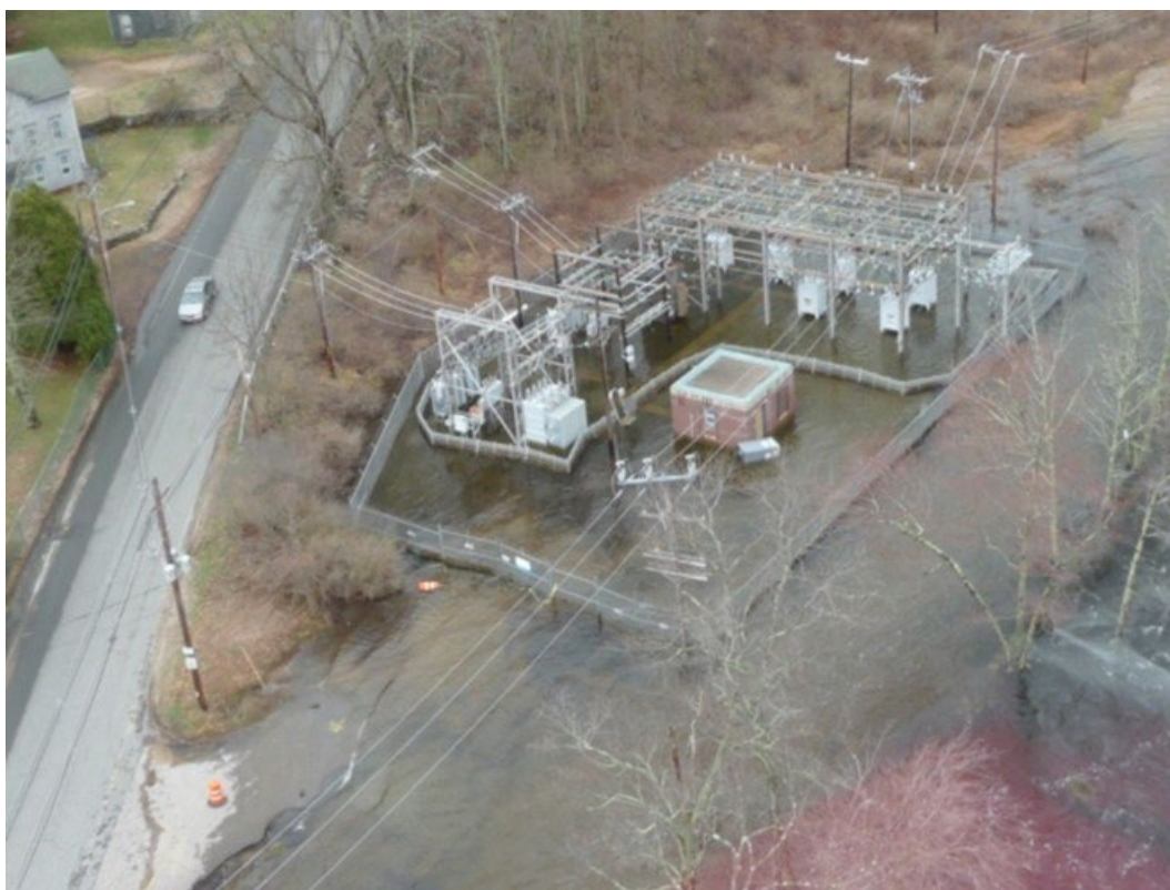
Figure 19: Flooded National Grid Substation
