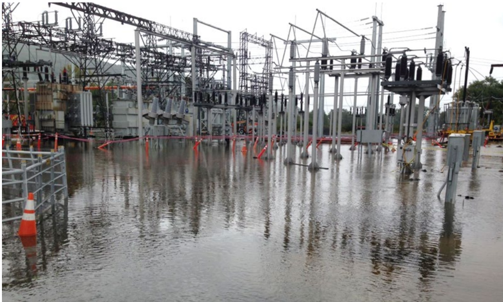
Figure 13: Adams, MA substation inland flooding in 2023
