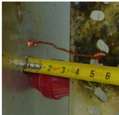
Figure 2-21 Arc initiation in the inverter cabinet for test 25
