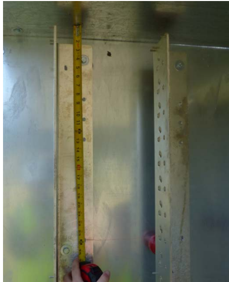
Figure 2-17 Arc initiation in the inverter cabinet for test 21
