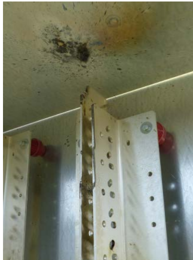
Figure 2-23 Arc damage for test 29
