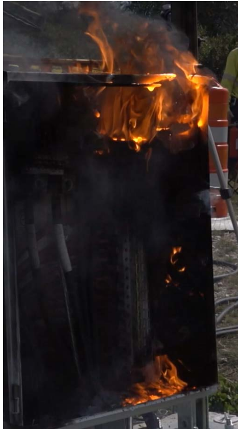
Figure 2-15 Damage from test 28
