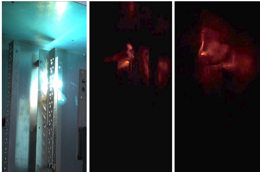
Figure 3-13 Arc flash and arc movement (infrared images) during a test #29 in the inverter assembly
