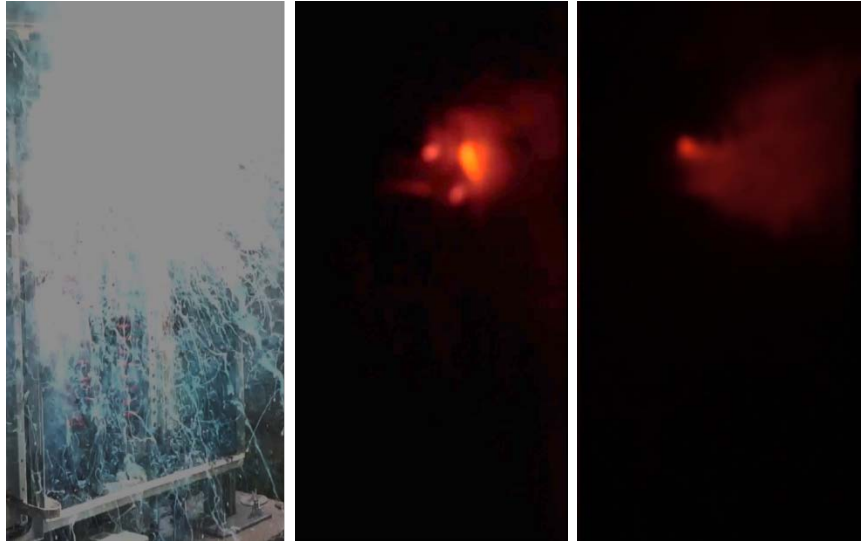
Figure 3-12 Arc flash and arc movement (infrared images) during a test #28 in the combiner box
