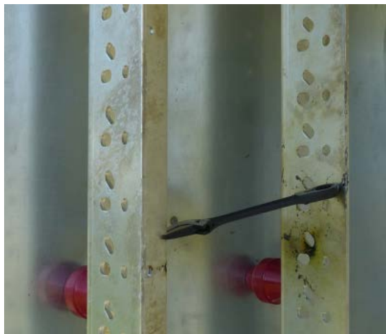
Figure 2-18 Arc initiation in the inverter cabinet for test 22
