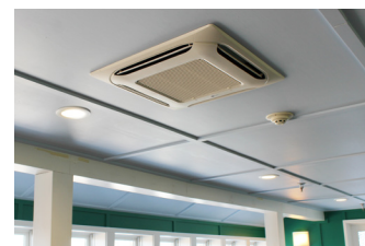
The Mass Audubon Joppa Flats facility utilizes ceiling vents throughout the building to evenly distribute heating or cooling.
